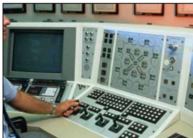
Figure 4: Control Panel at Nuclear Plant – Control Threats
